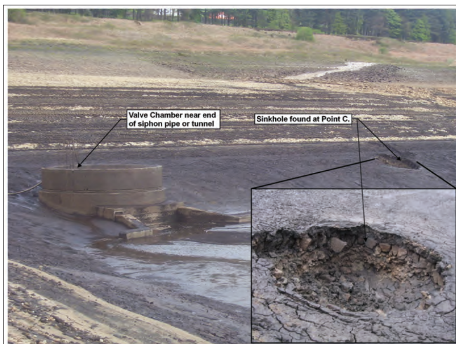
Figure 14. After the reservoir was drained, a sinkhole was found at Point C.
